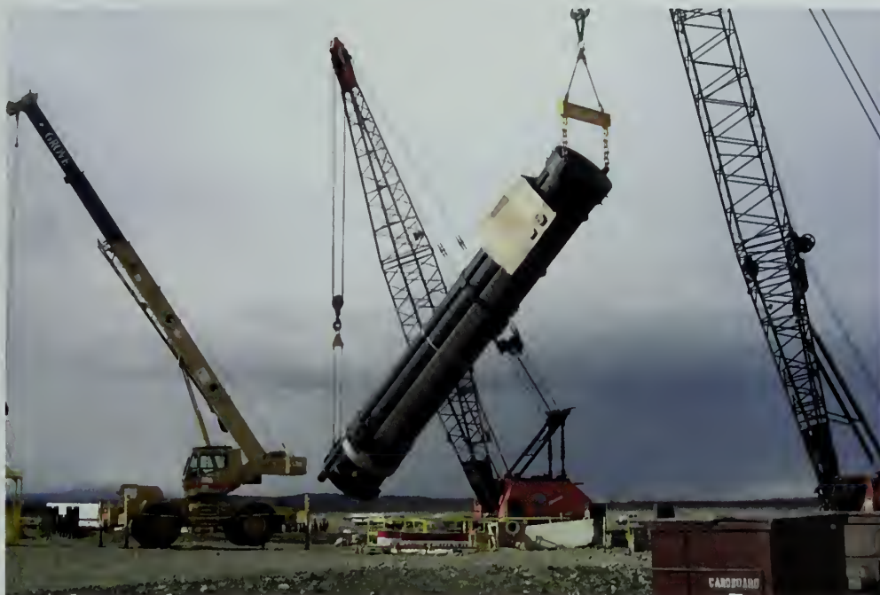
Fig. 6-20. Installation of the first of six Ground-based Midcourse Defense missile silos at the GMD Testbed at Fort Greely, Alaska in 2003. The 75-foot long silo weighs 130,000 pounds.
